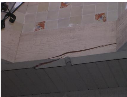
Fresh Split in Beam 12.20.09
